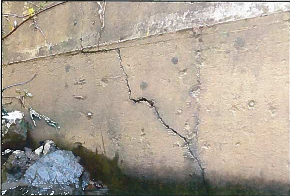
Photograph No. 17: View of Shear Crack above the Water Line on West Wingwall of Abutment 2, Looking East.
