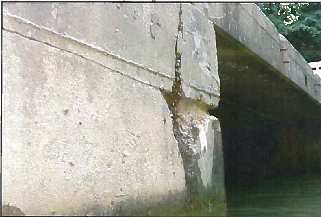
Photograph No. 18: View of Spall on West Wingwall of Abutment 2, Looking Southeast.
