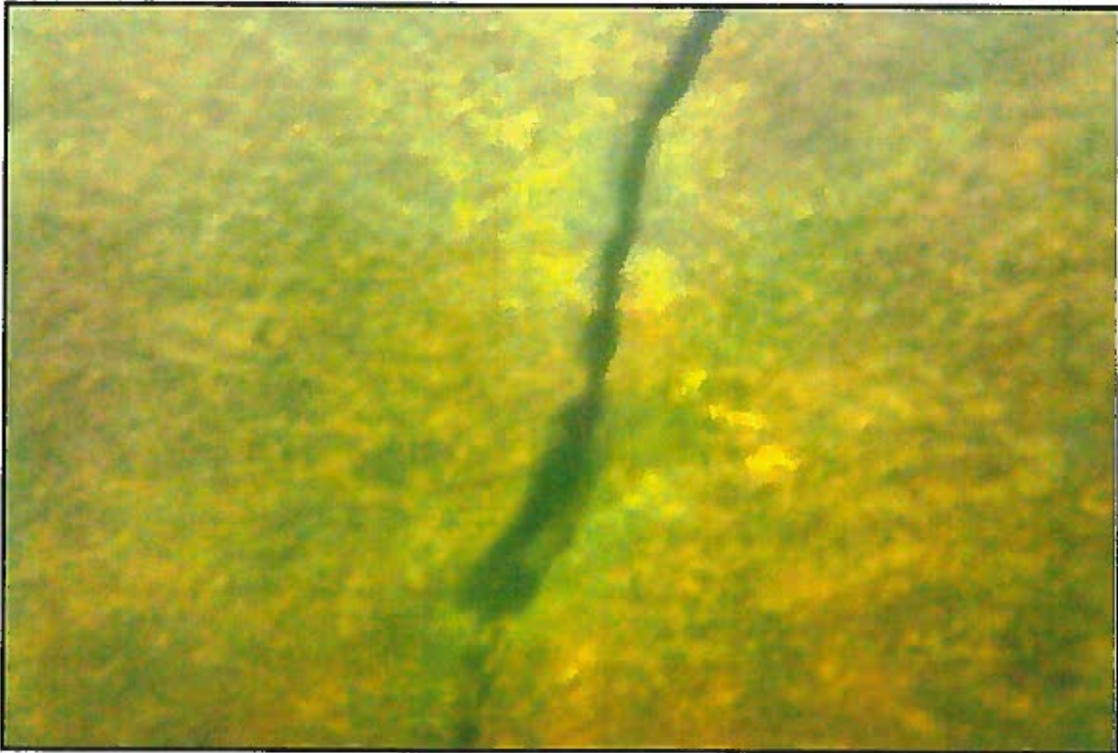
Photograph No. 15: View of Shear Crack below the Water Line on East Wingwall of Abutment 2, Looking West.
