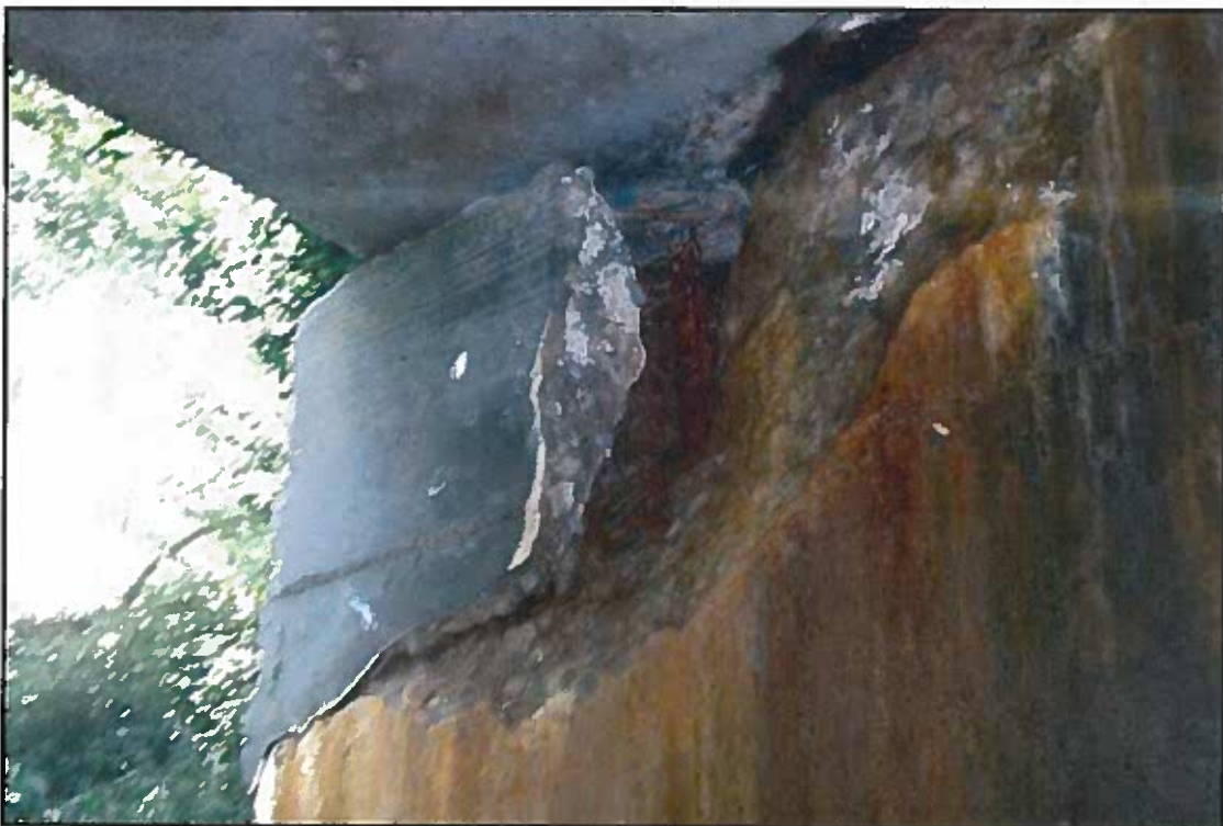
Photograph No. 10: View of Failed Concrete Repair at Upstream Corner of Abutment 1, Looking South.
