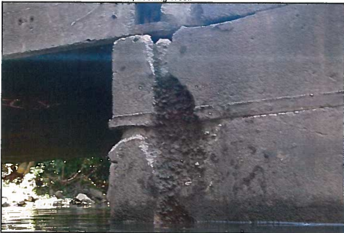
Photograph No. 16: View of Spall on East Wingwall of Abutment 2, Looking Southwest.
