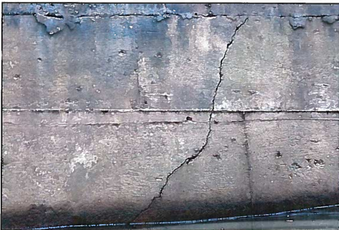
Photograph No. 14: View of Shear Crack above the Water Line on East Wingwall of Abutment 2, Looking West.
